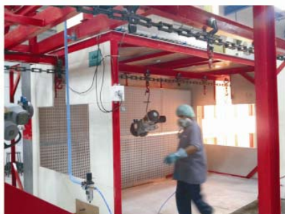
Spray Paint Booth
