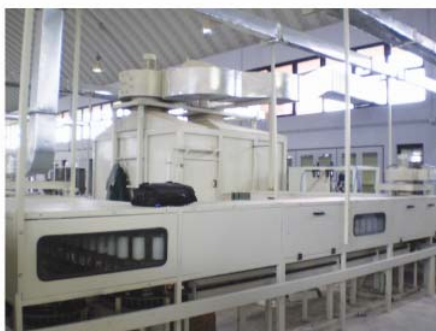
High speed automatic paint shops ( in pics: high speed line for filters )
