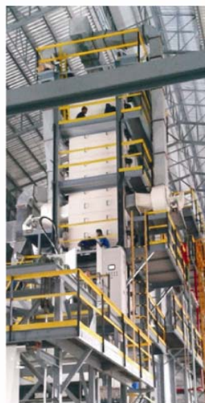
Tower dryers for Glass-fibers / Teflon curing / Tyre cords
